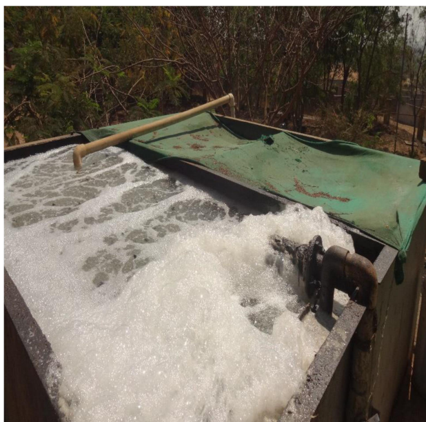
Liquid Waste Management Plant
