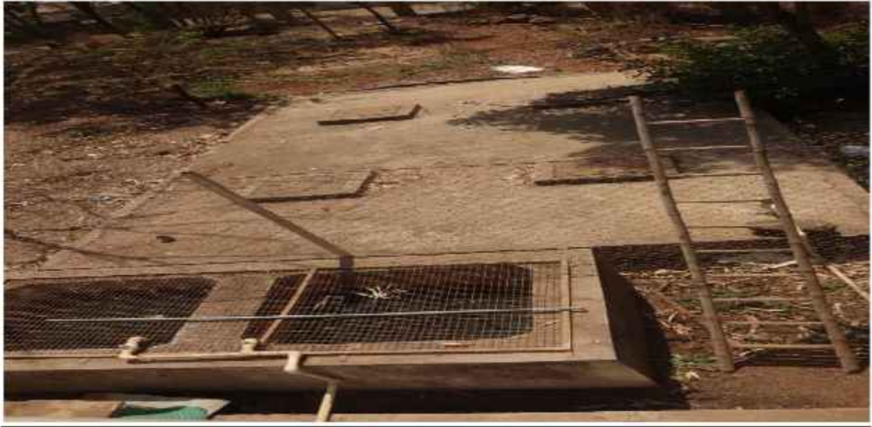
Septic Tank having capacity 1.25lakh litres
