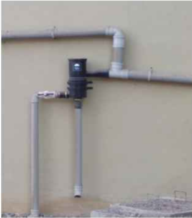
Filter at P1 Building
