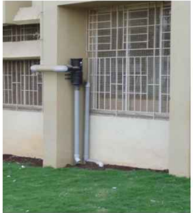
Filter at P2 Building
